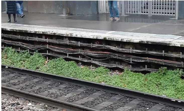
Figure 7: Cable congestion under platforms
